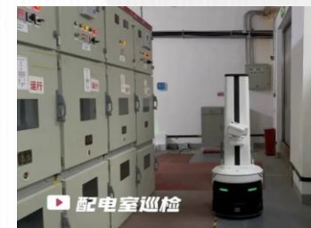
Key Space Inspection Robot
