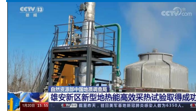
Gravity heat pipe in Xiong'an New Area
