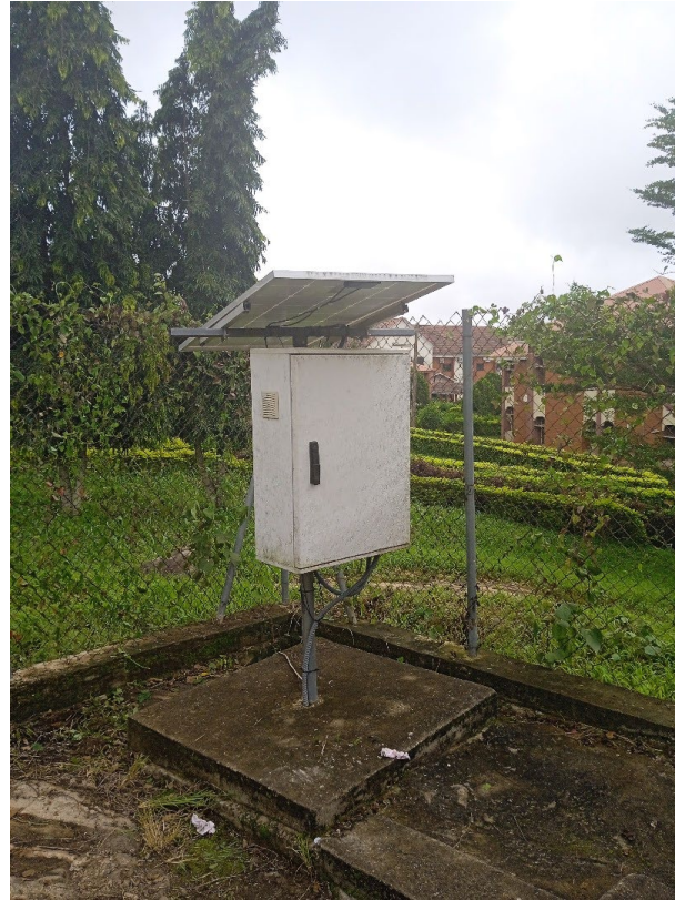
CORS Receiver, Comms and Power unit
