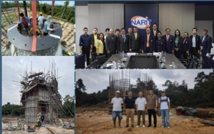
MoU Signing Walailak Univ. - NARIT, 2 Sep 2024 Constructing the Nakhon Si Thammarat station.
